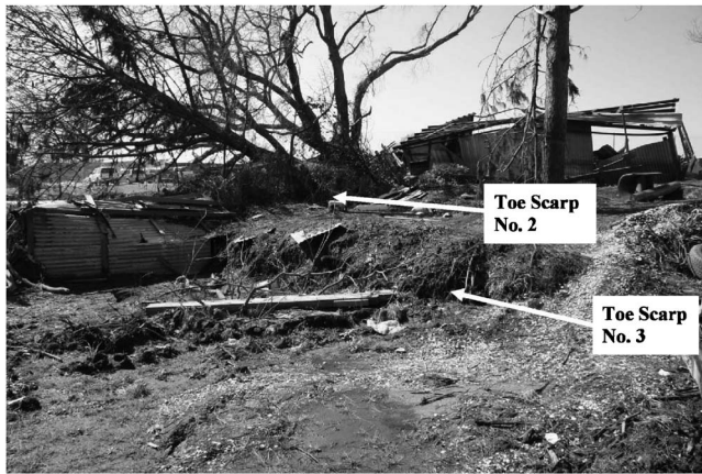
Fig. 6. View of Toe Scarp Nos. 2 and 3 at the inboard edge of the lateral translational failure at the 17th Street drainage canal
